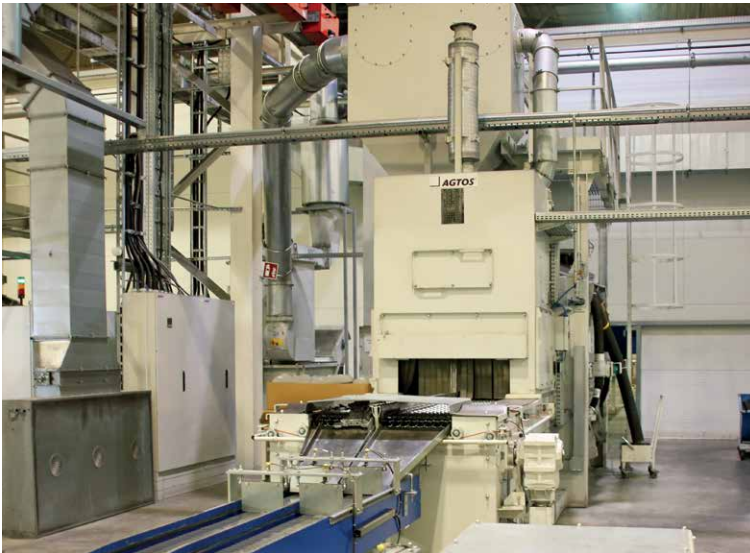
Discharge side of one of the shot blast machines installed at ae in Gerstungen
